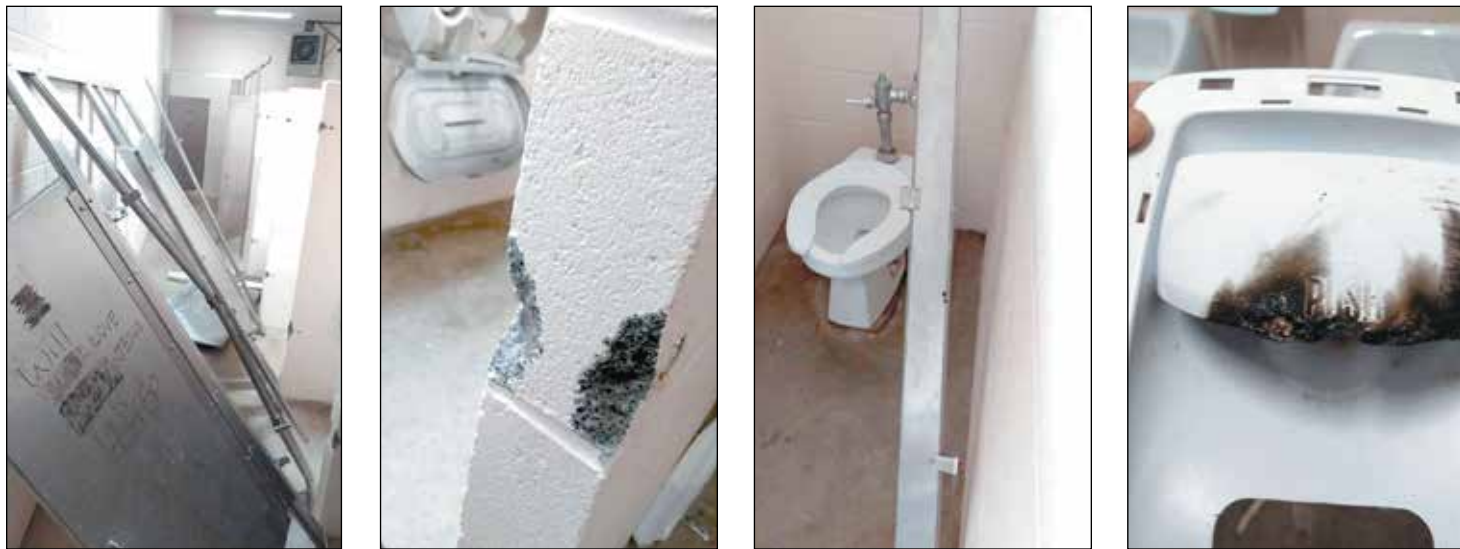
COSTLY DAMAGE – One night of vandalism has resulted in a repair bill exceeding $7,300 for the Camden City Park.
